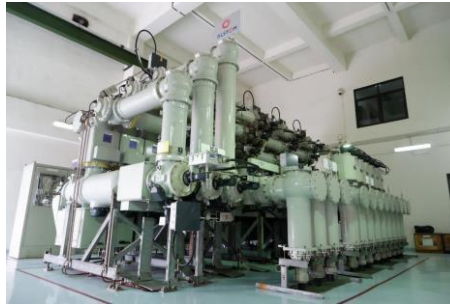
Gambar 1 GISTET (Gas Insulated Switchgear Tegangan Ekstra Tinggi)
