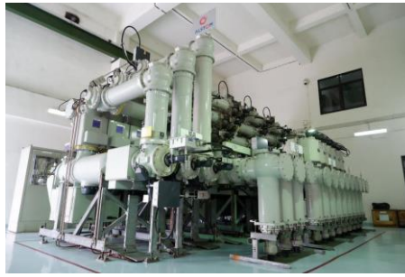
Gambar 1 GISTET (Gas Insulated Switchgear Tegangan Ekstra Tinggi)
